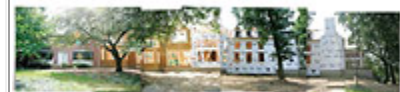
Four photos pieced together show the construction under way to combine two homes in Clintonville.
